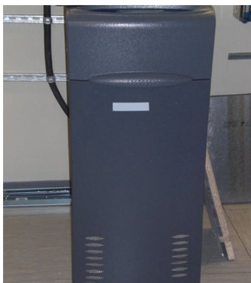
The Culprit: the UPS System
