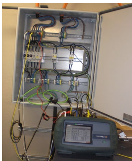
Mavowatt 40 in Action: Measurement at the UPS System's Distributor
